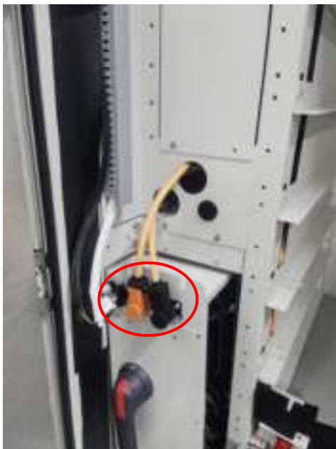
B+ and B- of tower voltage
