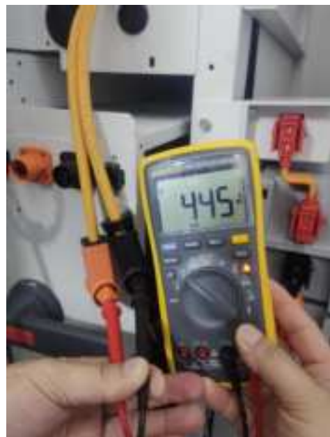
Measurement of tower voltage
