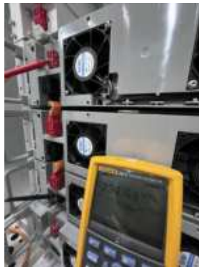
Multiple Module Measurement
