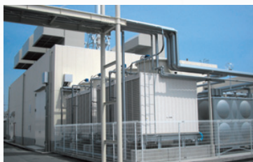
The cogeneration system installed through the ESCO.
