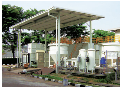
The upgraded water treatment facilities
