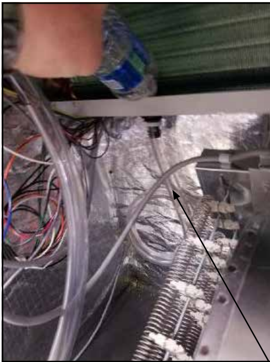
Evaporator Drain Pan Left Side Drain Hose
