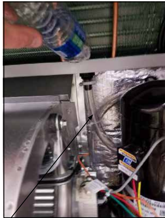
Evaporator Drain Pan Right Side Drain Hose
