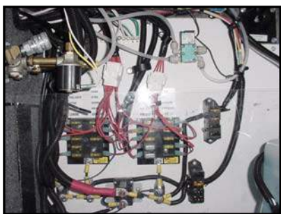
Figure 7-4. 12 VDC Fuse Panels
