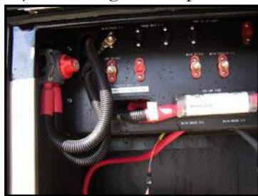
Figure 7-7. Rotary Switch to Disconnect Engine Battery
