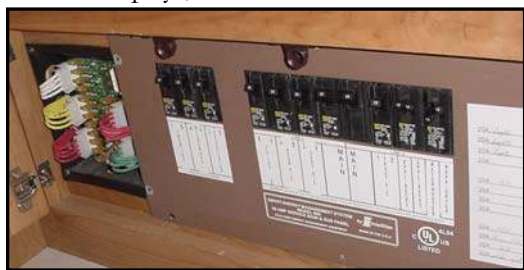
Figure 7-3. Circuit Breaker Box
