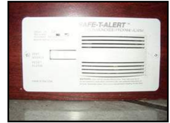
Figure 3-8. CO/LP Gas Detector
