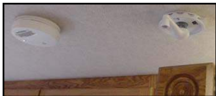
Figure 2-8. Smoke Detector (Left)
