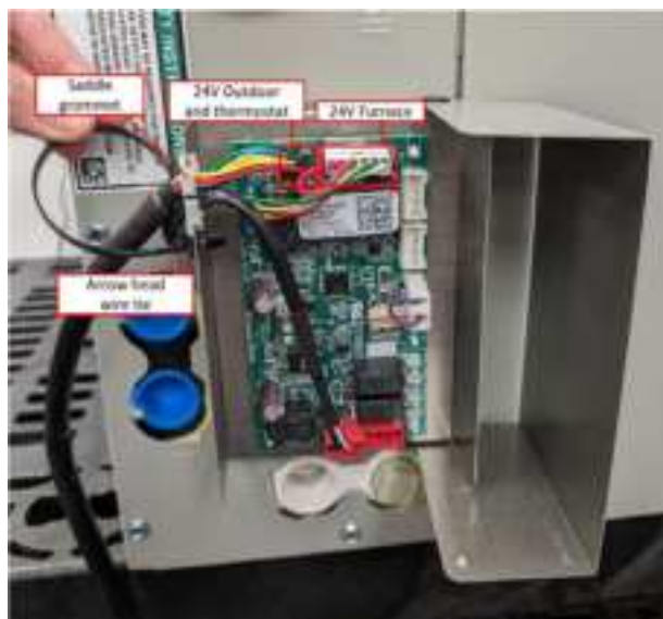
Figure 12: 24VAC harness connection to MCB
