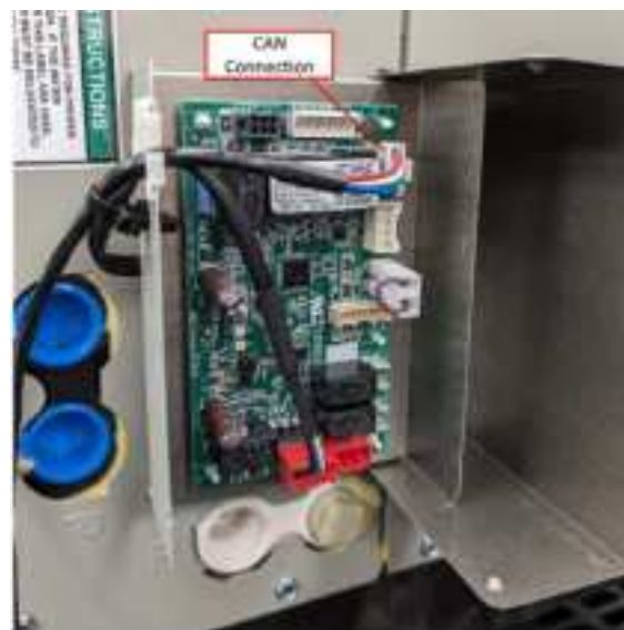
Figure 13: Comm/Link harness connection to MCB
