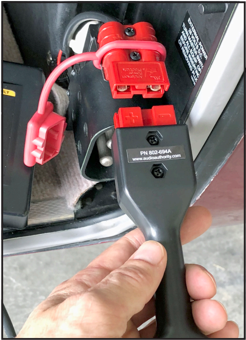
Figure 5. Finished installation example.
