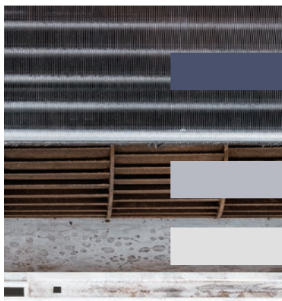
No Dual Barrier Coating
