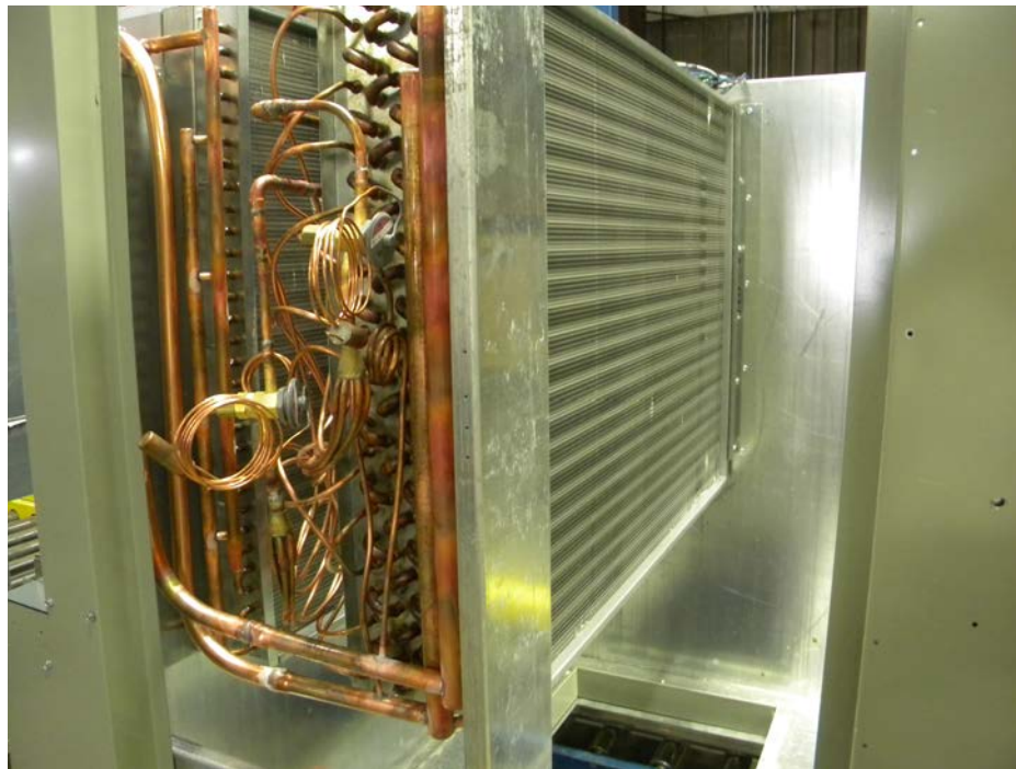
Figure 79. Evaporator and reheat coil
