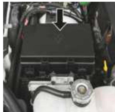
Power Distribution Center
