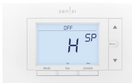
Humidification Control at the thermostat
