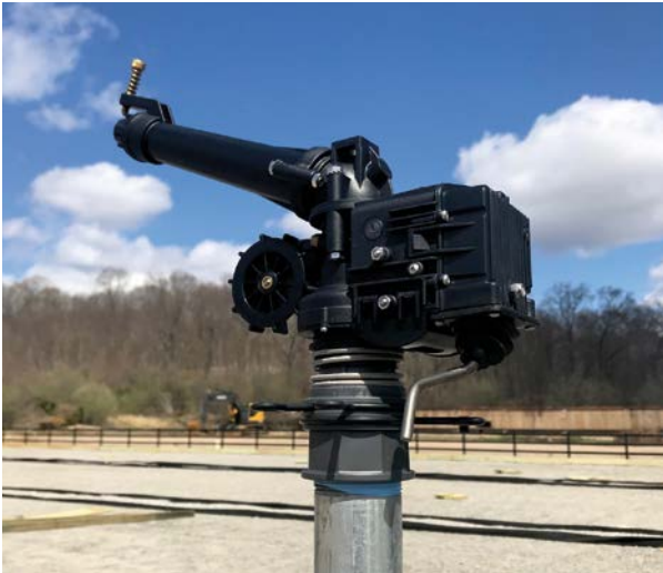
ST-1200-BR Rotor Installed
