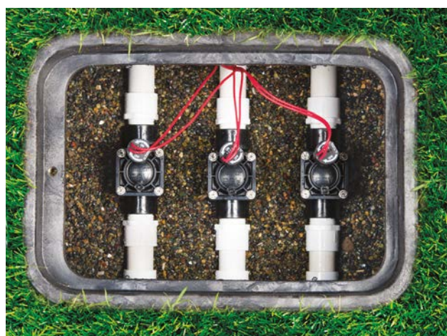
PGV-100G Valve Installed
