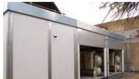
MCP with Dual Chillers Inside
