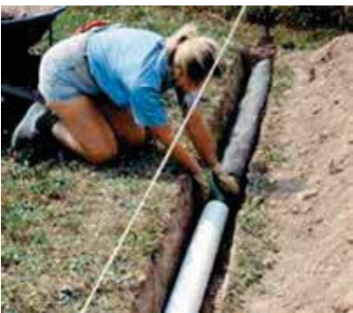
Figure 275: Underground Refrigerant Piping.
