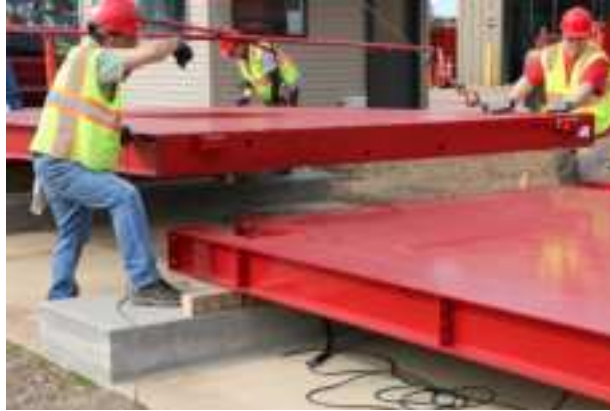
Figure 3-5. Module B Installation
