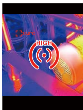
High Temp Alarm
