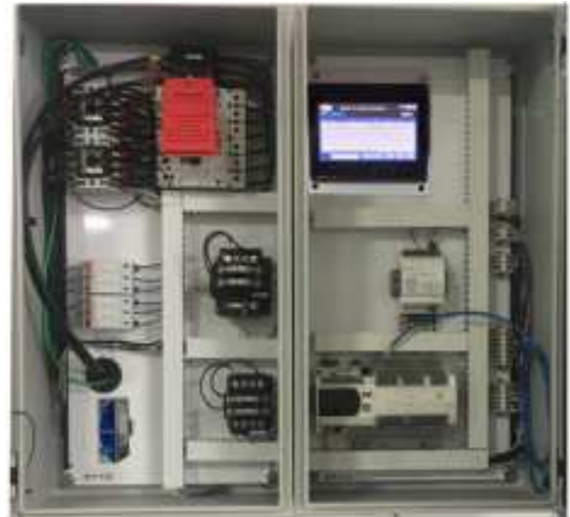
Figure 22. Module electrical and control panel
