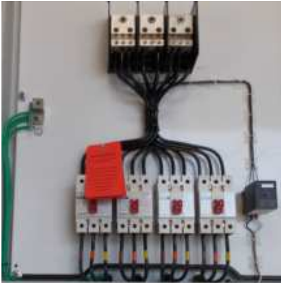
Figure 21. Power distribution panel
