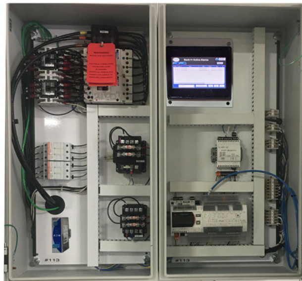
Figure 22. Module electrical and control panel
