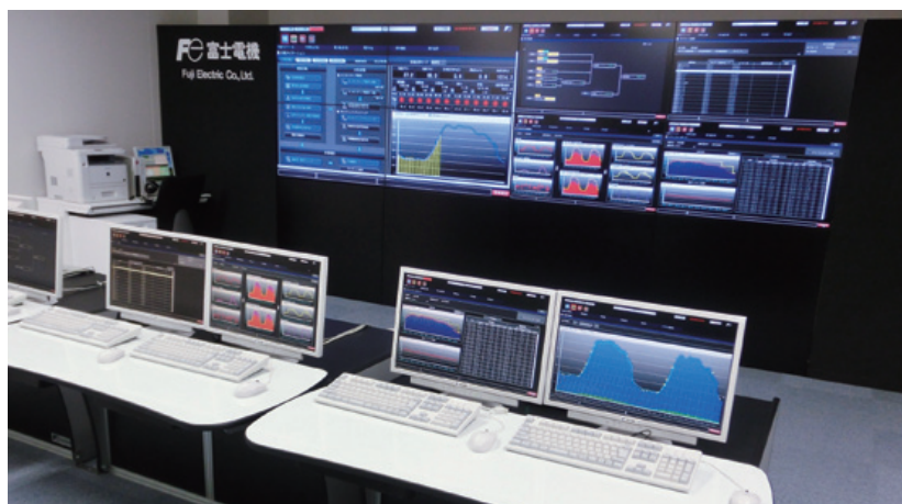
Cluster Energy Management System (CEMS)
