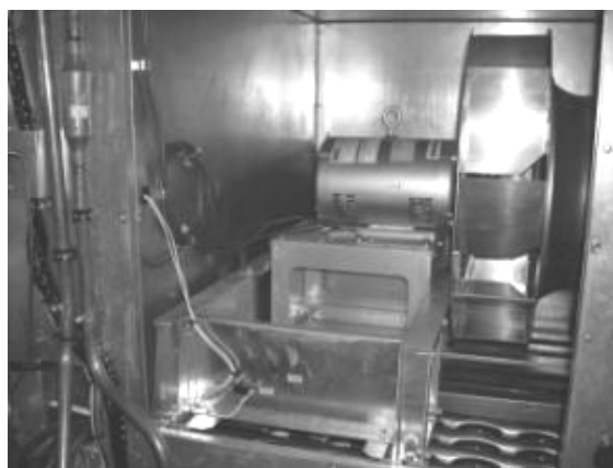
Figure 38 - 11-25 and 30 ton Supply Fan
