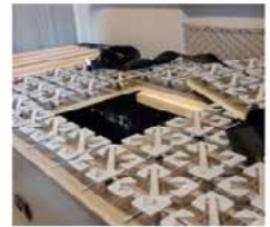
Water heater Bypass
