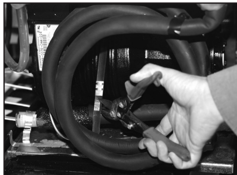
Cutting band that is around compressor
