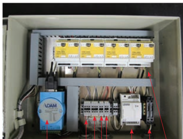
Figure 2: Interior of Enclosure
