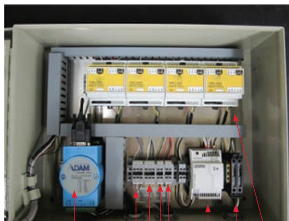
Figure 2: Interior of Enclosure
