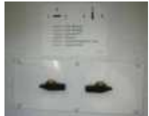
Fig. A -Water Valve Controls
