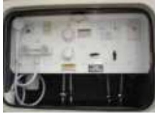
Fig. B - Utility Center
