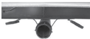
Black/Grey Tank Drain and Valves
