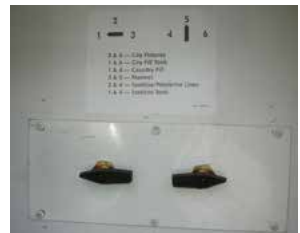
Fig. A -Water Valve Controls
