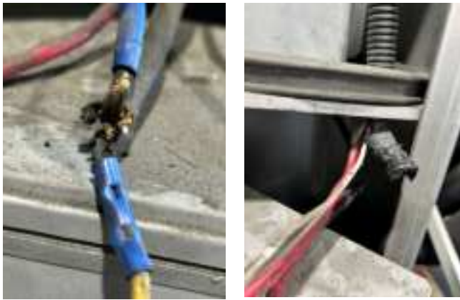
Fig. 1 - Examples of damaged wiring insulation
