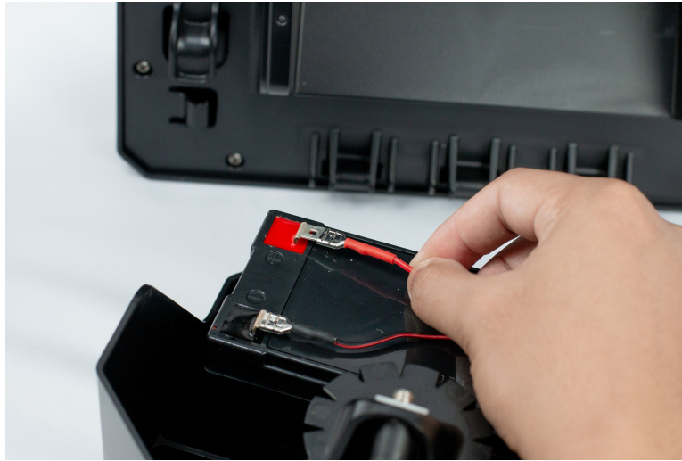
Figure 9: Connecting the Battery Terminal
