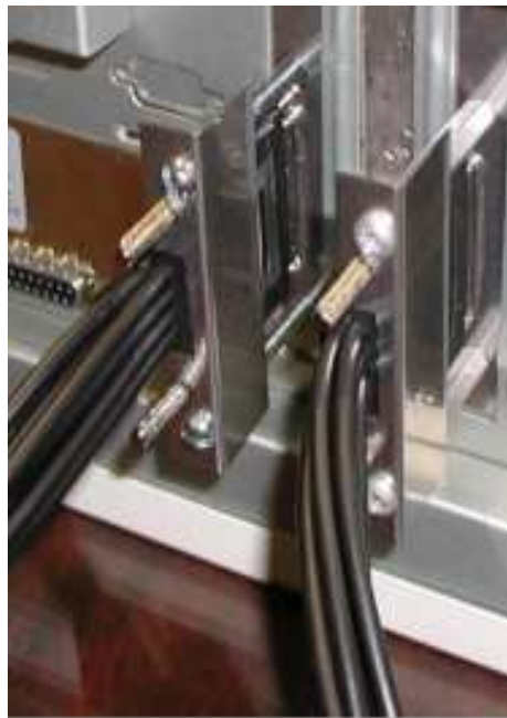
Figure 2-1: Installed Cards with Stability Bracket Accessories
