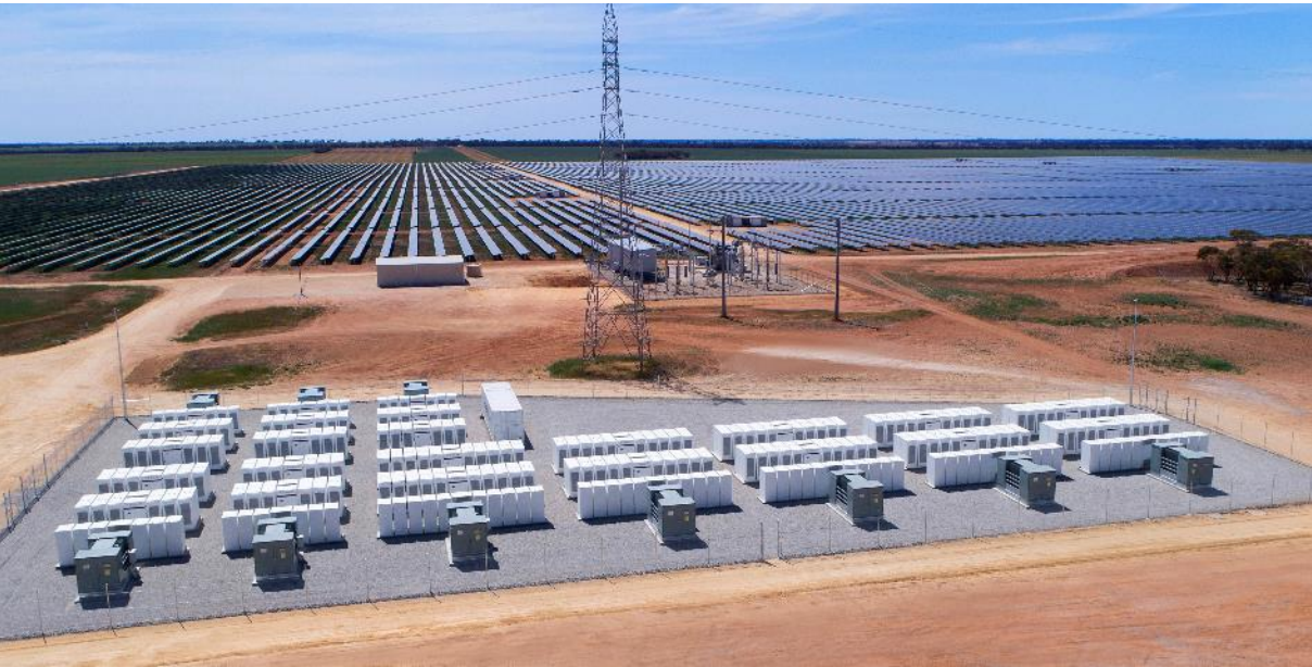
Commercial Solution: Solar and Storage
