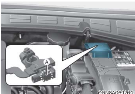
[A] : Battery sensor
