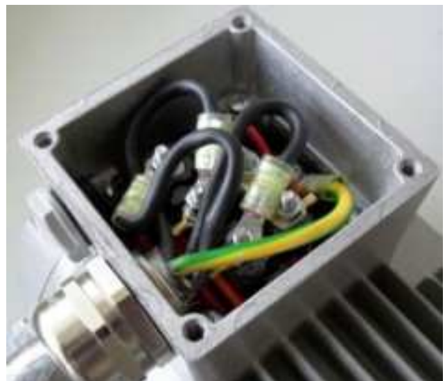
Fig. 30: Wiring on the motor connection box
