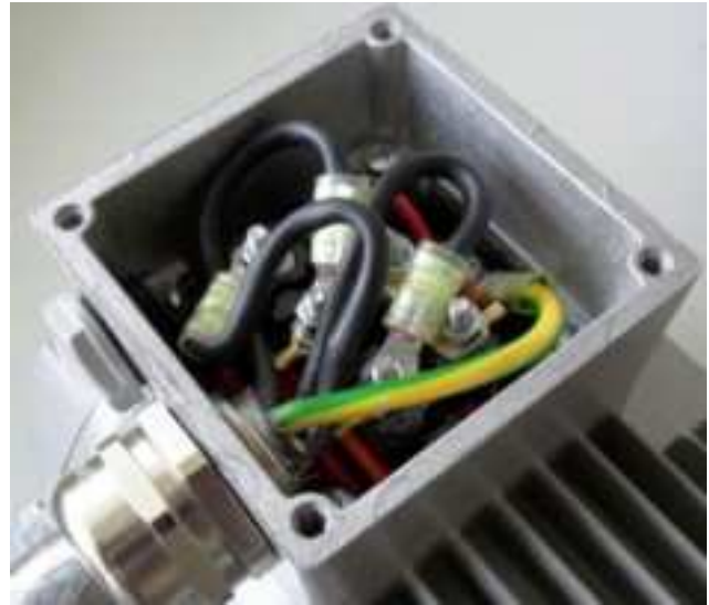
Fig. 23: Wiring on the motor connection box
