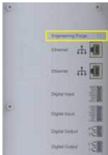
Figure 3-13. Engineering Purge push-button on Connection panel
