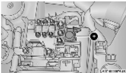
Positive Battery Post
