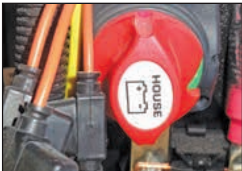
Figure 8-4: House battery disconnect panel switch
