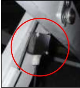
Picture 16 (up limit switch)
