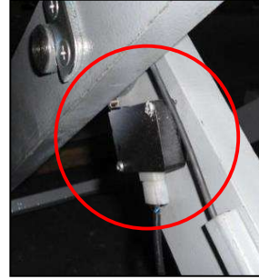
Picture 17 (lower limit switch)
