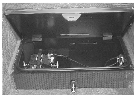
House Battery in Top Entrance Step
