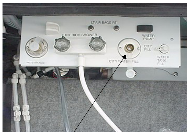
City Water Connection
