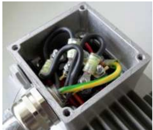
Fig. 32: Wiring on the motor connection box
