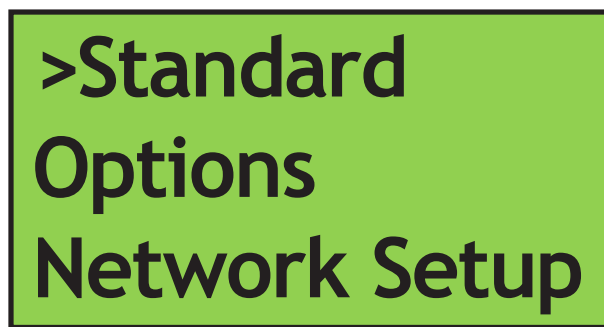
FIGURE 5 - Commissioning View: Second Level Menus
