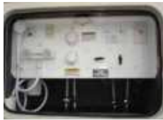
Fig. B - Utility Center
