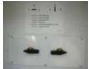
Fig. A -Water Valve Controls
