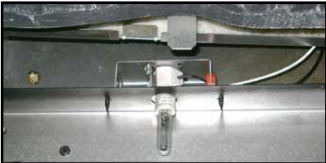
Figure 11.10 Ember Light Bulb Installed
