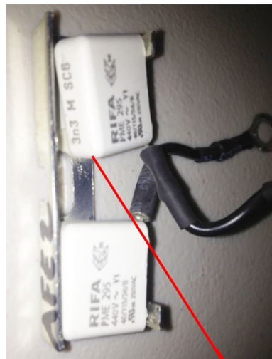
Close-up View of Common Mode Capacitor Assembly
