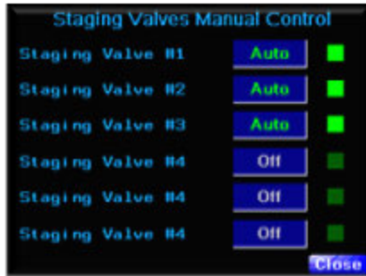
Figure 28. Staging valves control screen
