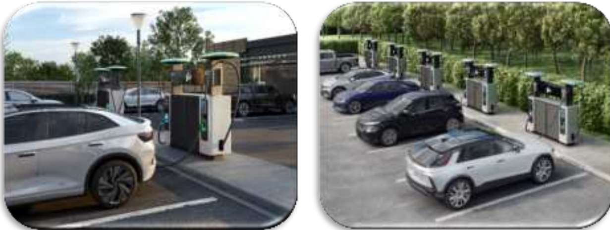
Figure 1 : Pull-In parking installation
