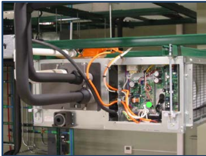
Fan Coil Control PCB
