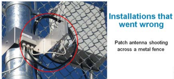
Figure 89 Patch Antenna Against a Metal Fence
