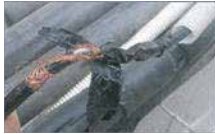
Example of Wiring Error.
