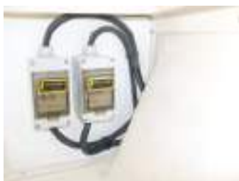
Breaker 220V - 32A (Reference 2)
