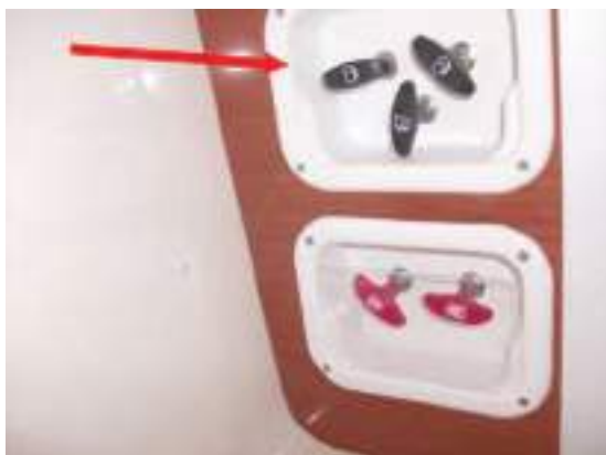
Remote pull switches - Supply tanks + generator
