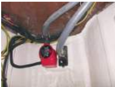
Electric bilge pump 12V - Engine compartment
