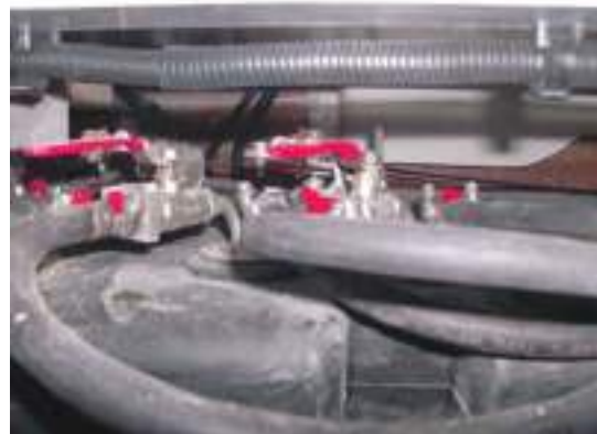
Fuel supply valve - Joining generator
