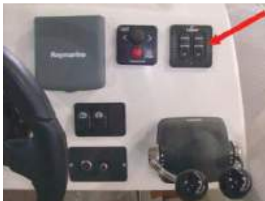
Control - Wheelhouse flying bridge
