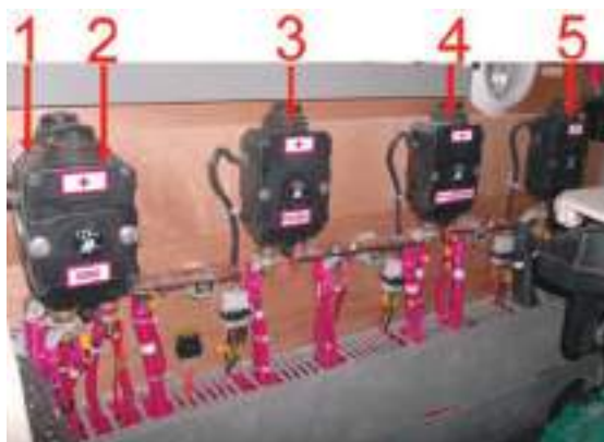
Electrical battery switches 12V - Location: Engine compartment
