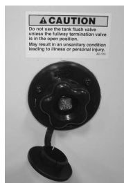
Tank Flush Inlet
