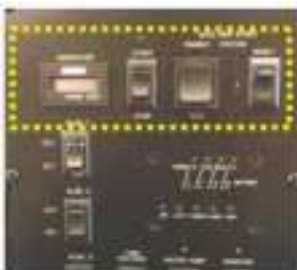
Command Center Panel
