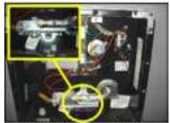
Fig 1: Water Heater Drain Plug
